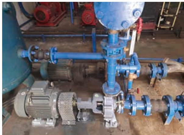
Water Pump Operation
